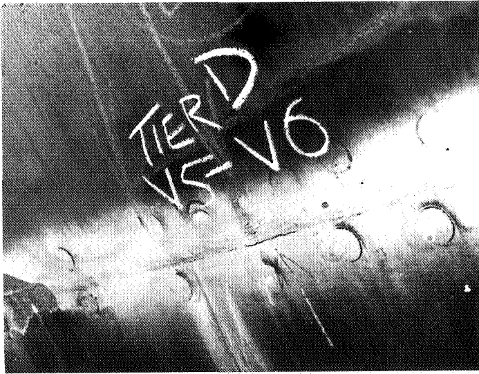
Figure 2. Crack in lower fusion line of horizontal weld in sphere.
